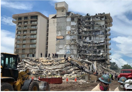
Fig.1. Illustration of the Champlain tower after its collapse [4].
